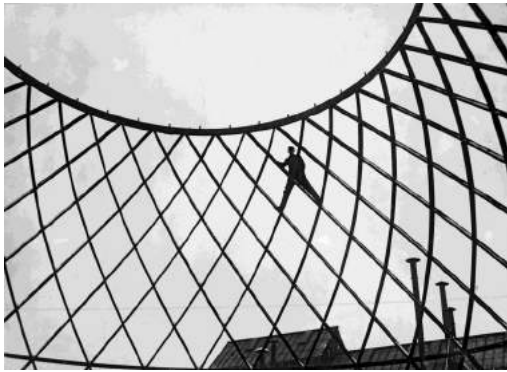
Otto Bartning Deutscher Reichspavillon building site , Milan, 1926 Unknown photographer © Atlantik Photos & Co
